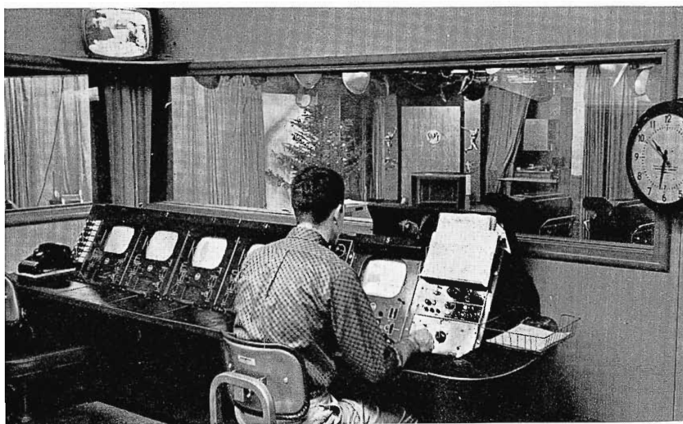
FIG. 14. Video Control. Five TM-6 Master Monitors are mounted in the console. The screen in the upper left displays the air signal. Video Supervisor John Raymond prepares for a switch.
